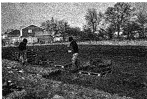
PLATE 2.1 Extracting turves by hand is not recommended. Turves should not be stacked or stored
