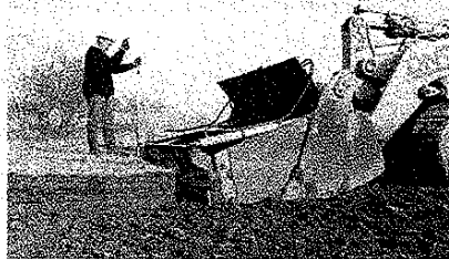
Plate 6.31 Specially adapted bulldozer bucket used for extracting pulverised fuel ash turves at Wilford Power Station
